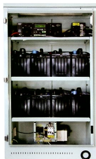
EXTERNAL UPS HOUSING
